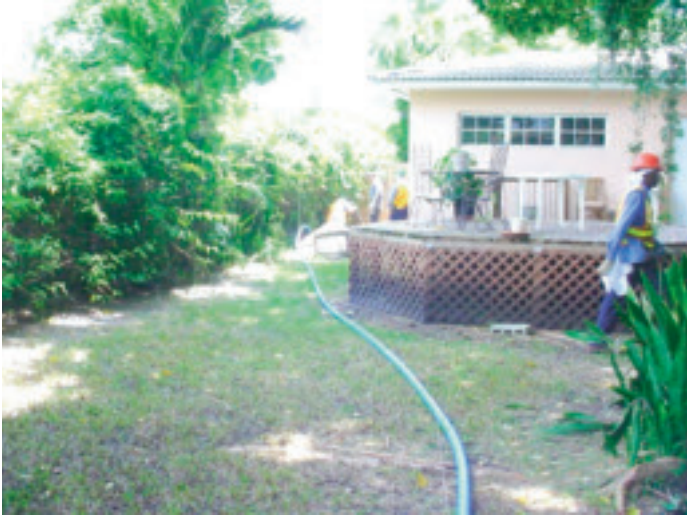
MIAMI, Fla. – A single long-run of 2-inch leak-free HDPE pipe is laid out, ready for installation. But instead of digging up this Miami-Dade Water customer's yard, the pipe will be snaked underground without any property destruction.
